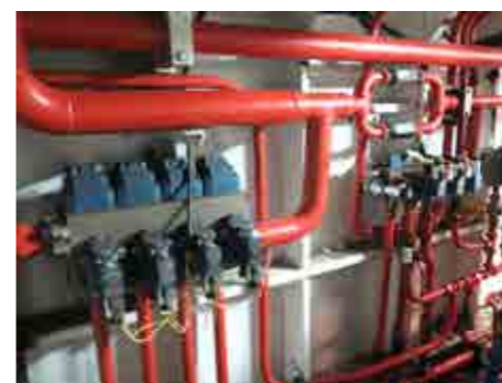
Left traverse winch manifolds
